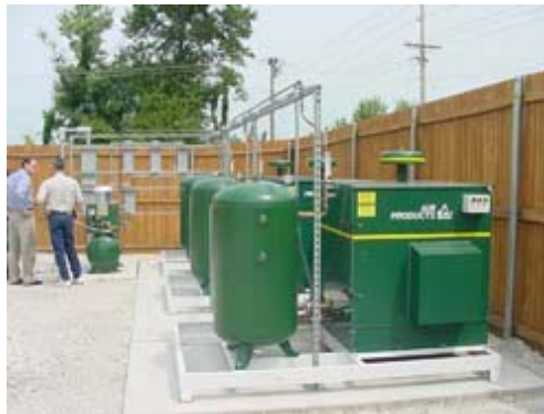
Fig.1a Modular oxidation system
