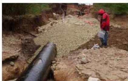
Fig. 6: The site where the aqueduct was broken by coseismic faulting
