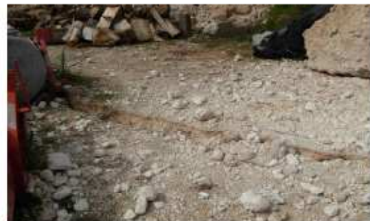
Fig. 5: The Paganica ruptures were traced in the ground, across buildings and concrete roads, more or less continuously, for at least 2.6 km with offsets up to 7-8 cm, which locally continued to increase in the following weeks
