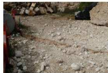
Fig. 5: The Paganica ruptures were traced in the ground, across buildings and concrete roads, more or less continuously, for at least 2.6 km with offsets up to 7-8 cm, which locally continued to increase in the following weeks.
