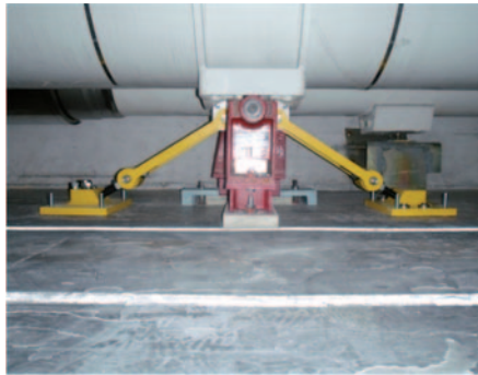
Fig. 6. – (Colour on-line) The reinforcement (yellow parts) on the floor supports of the SSS with vacuum barrier.
