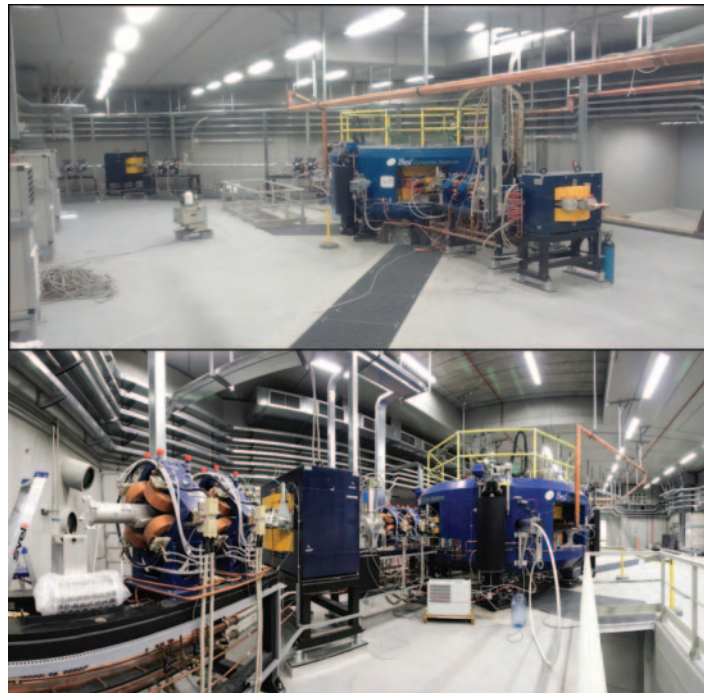
Fig. 2. – Views from the SPES building area where the B70 BEST cyclotron is installed. In the lower picture the beam line towards the RIB production is in the foreground.
