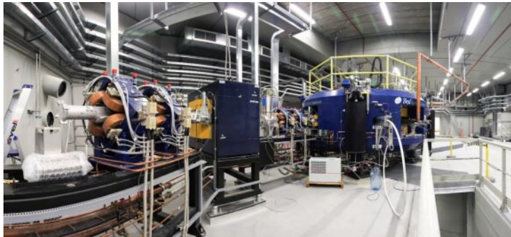
Fig. 2. – Views from the SPES building area where the C70 BEST cyclotron is installed.
