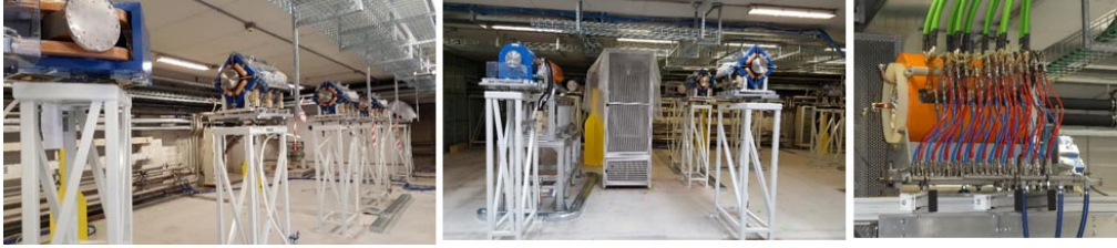
Fig. 3. – The ADIGE Installation phase: on the left: transport line towards the RFQ; center: Optical elements around the MRMS; on the right: Cabling the Charge Breeder.
