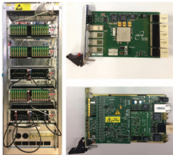
Fig. 6. – Left: MEG II rack. Each rack contains up to 10 crates, each crate contains 16 WDBs and a TCB. Top right: picture of a TCB. Bottom right: picture of a WDB.
