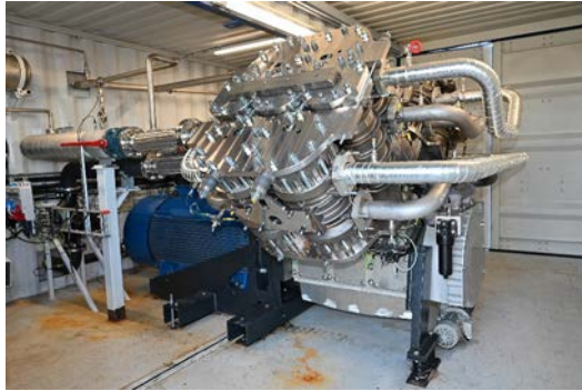
Figure 1. HoegTemp heat pump installed at IVAR biogas facility, Stavanger, Norway.
