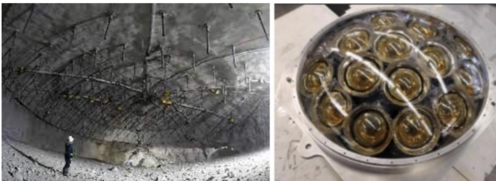
Fig. 4. – HK dome excavation at July 2023 (left) and one of the nPMT's (right).
