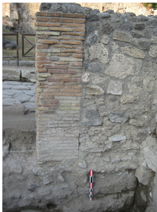
Fig. 21. The rebuild of the southern side of the façade with a brick quoin.
