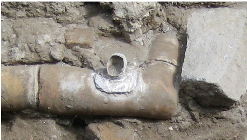
Fig. 39. The lead joint within the terracotta pipe that came from WF 464.
